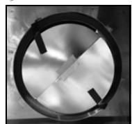
Black Tape on Damper
